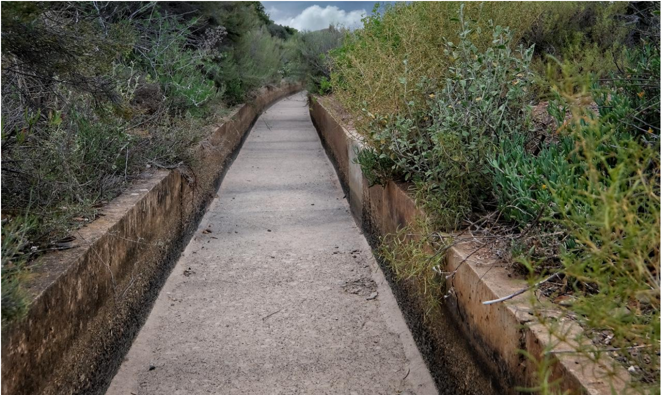
Construction has stood the test of time
