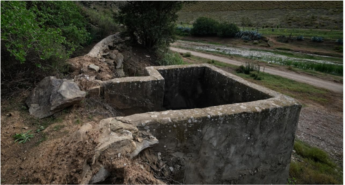
An abandon sluice gate
